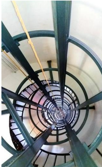
The prefabricated glass tube through the staircase well which will accommodate the lift.
