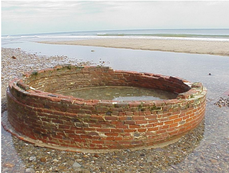
Foundation of the Center 'Sister' Lighthouse courtesy of the National Parks Service
