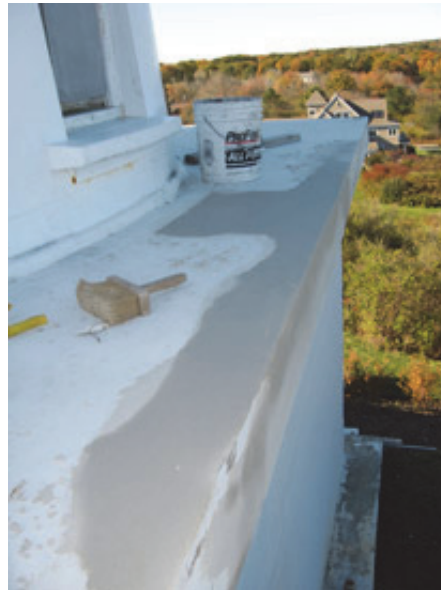
(Photo by Bob Trapani, Jr.) Ken Morse applies new cement to repair spalling damage
