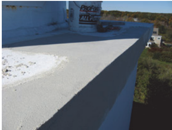
A close-up view of the repair work by J.B. Leslie Masonry on the east side of the concrete overhang
