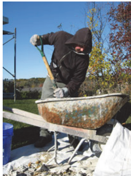
(Photo by Bob Trapani, Jr.) Jake Johnson works to mix a round of cement
