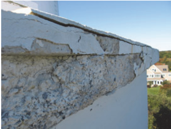
A close-up view of the deterioration that occurred to the light's concrete base on the east side
