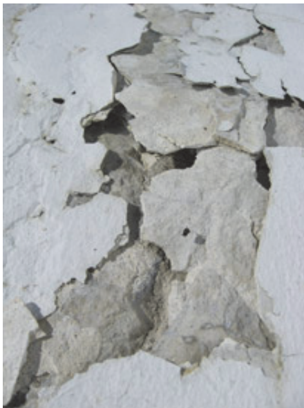
(Photo by Bob Trapani, Jr.) A close-up view of failing cement on the top of the base
