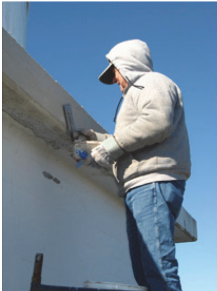
(Photo by Bob Trapani, Jr.) Ken Morse applies new cement to repair spalling damage
