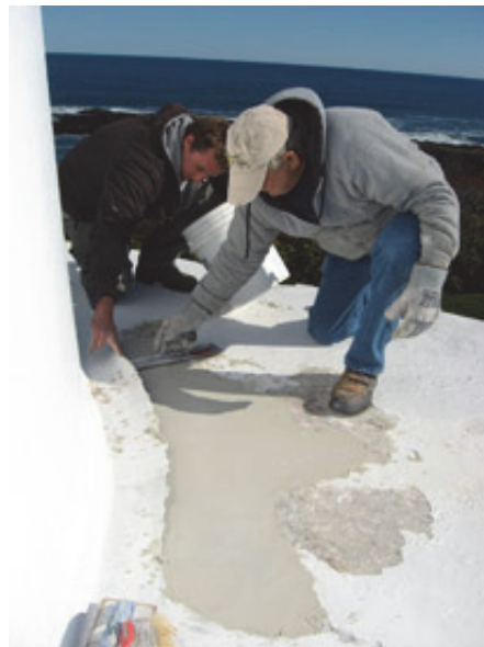
(Photo by Bob Trapani, Jr.) Jake Johnson and Ken Morse repair a top section
