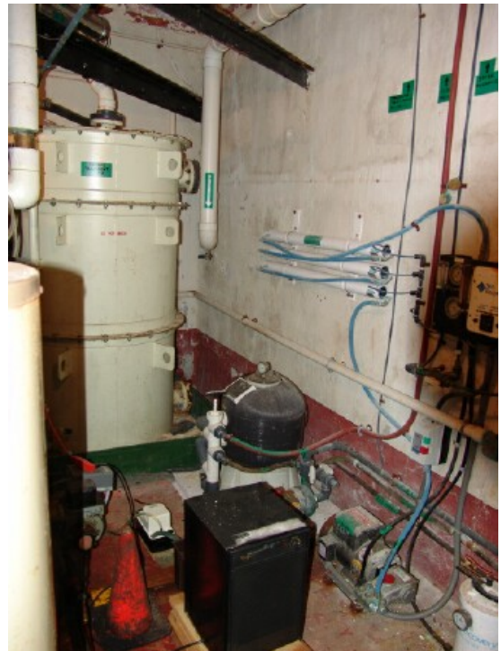
Water filtration equipment in the basement
