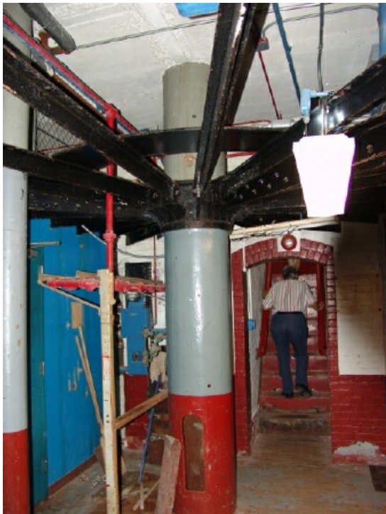
Steel girders fan out from the center post to strengthen the structure
